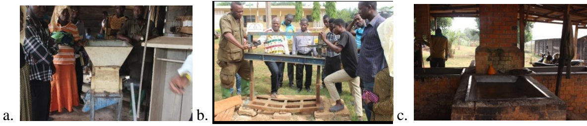
Figure 4: Cassava processing plant a. Grater b. Presser c. Gari roasting set up at Duayaw Nkwanta Prison Camp
